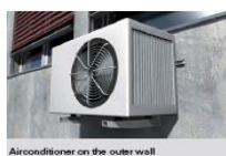
Airconditioner on the outer wall
