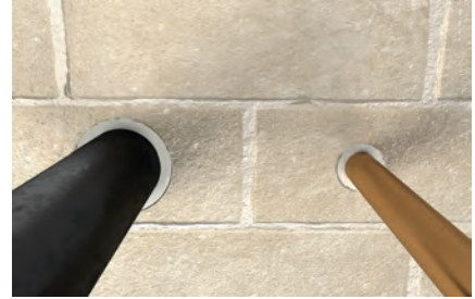
Non combustible services
