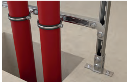
Waste water pipe
