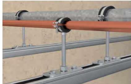
Baseplate on installation channel
