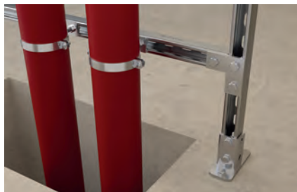
Waste water pipe
