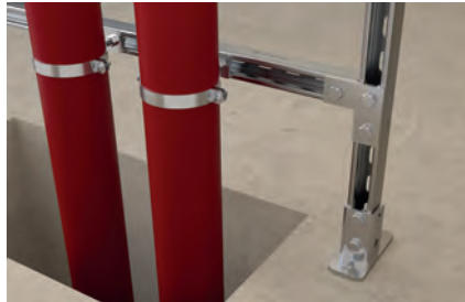
Waste water pipe
