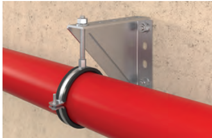
Heavy drainage pipe under angle bracket
