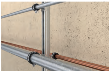
Lateral pipe mounting at channel
