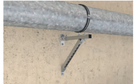
Spiral airduct on cantilever
