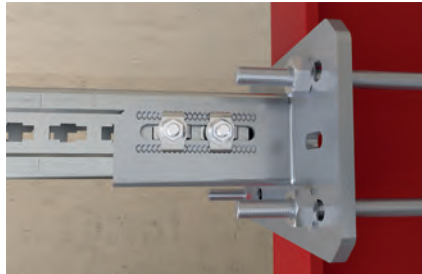
U-rack at profile traverse
