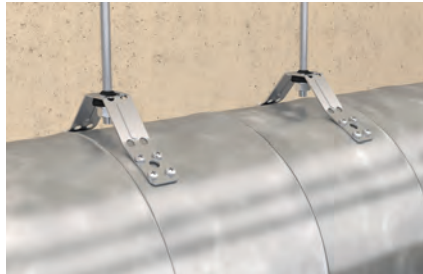
Spiral duct pipe with sound insulated hanger
