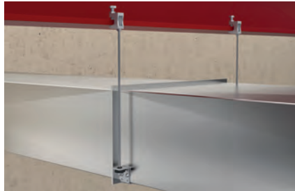
Airduct under steel beam with beam clamp
