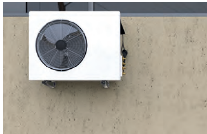
Airconditioner on the outer wall
