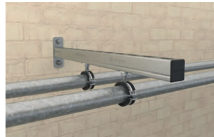
Pipelines on cantilevers
